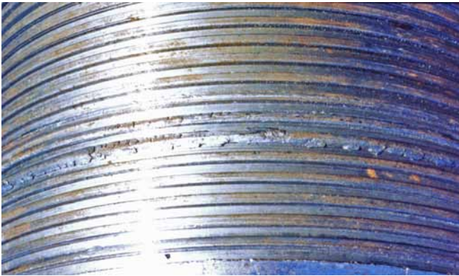
FIGURE 19. Galling on pipe thread.
