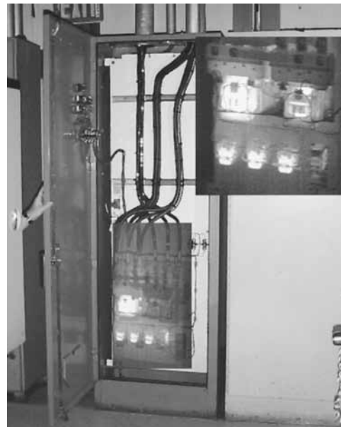
FIGURE 12. Infrared thermography of automatic transfer switches for emergency diesel generator. Hot spots appear bright in thermogram (inset).
