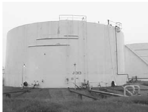
FIGURE 2. Aboveground storage tank for petroleum products.
